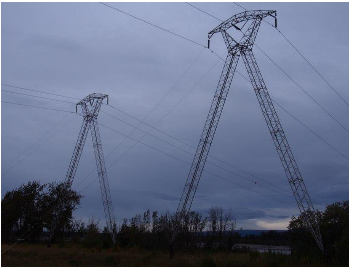
BELUGA POWERPLANT TRANSMISSION LINE — Susitna River: From Glaciers to the Sea. Leg 3: To the Sea — Get Photo (/photos/beluga-powerplant-transmission-line/)
